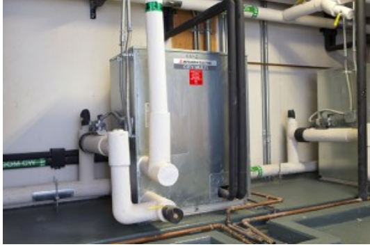
The mechanical room in the Elliot and Stoddard Halls houses three Mitsubishi Electric water-source heat pumps.
